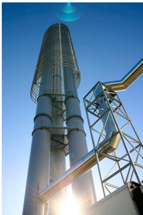
Clinical waste incinerator exhaust stack
