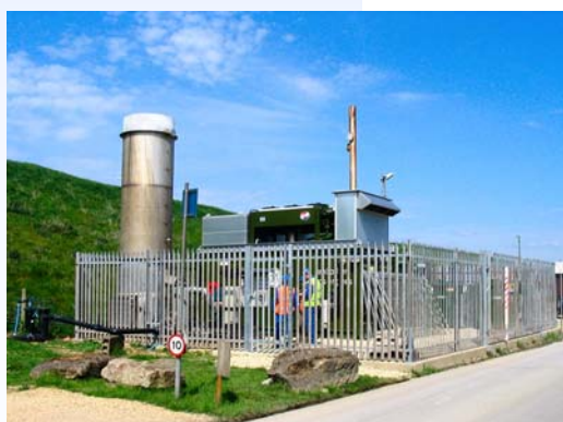
Gas engine at Wingmoor Quarry Landfill
